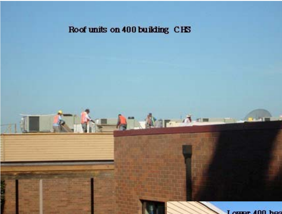
Lower 400 heating/cooling unit
